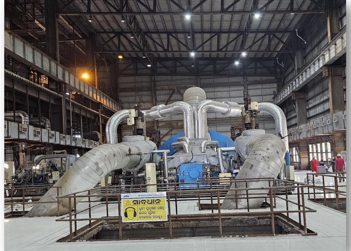
Unit 1 Turbine Generator set
